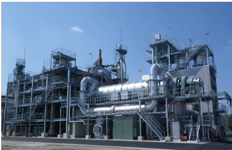
< Sewage-Sludge-to-Fuel Conversion conversion facility >
