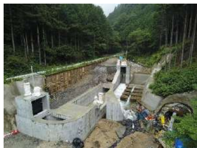
Seinaiji hydro power (current status)
