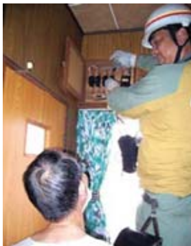
Power distribution engineering service representative checks the wiring in an elderly person's home
