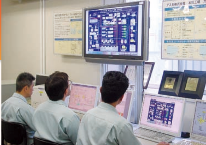
Monitoring room at ASMO Co., Ltd.
