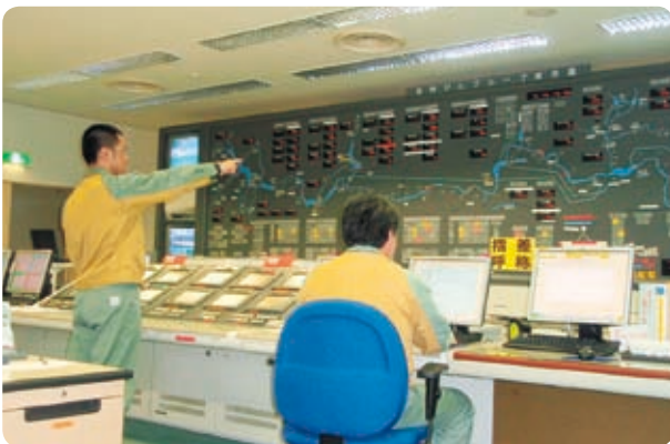
The dam being monitored at Akigami Dam Control Office
