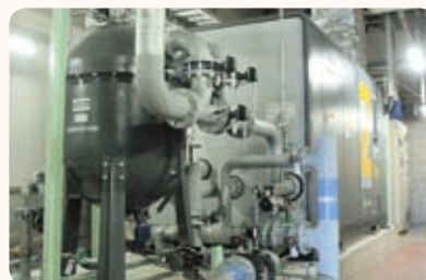
One of the world's largest-class screw inverter compressors and adsorption dryer
