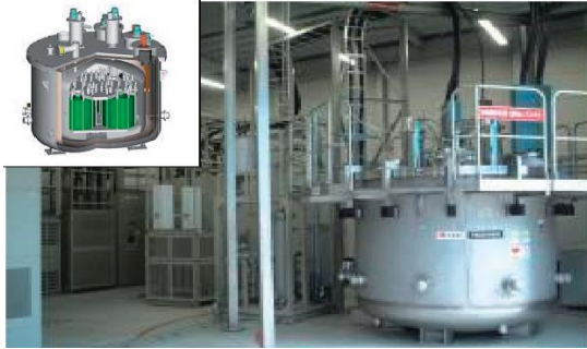
Verification test of SMES (5,000kW / 1 second)
