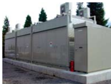
An uninterruptible power supply system incorporating a high-voltage, high-capacity double layer capacitor
