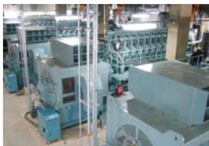
On-site energy facility
