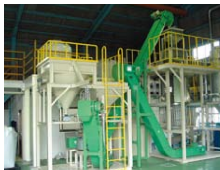
Development of equipment for CFC destruction
