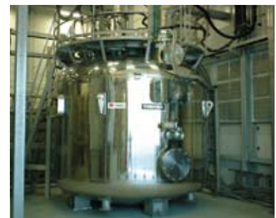
Verification test of SMES (10,000 kW/second compensation)
