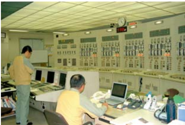
Central control room
