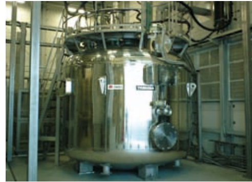
Verification test of SMES (10,000 kW/second compensation)
