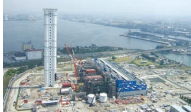
Shin-Nagoya Thermal Power Station Group No.8
