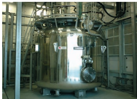
Verification test of SMES (10,000 kW/second compensation)
