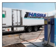
Electricity supply station offering external power source to cut truck idling
