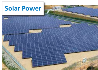
Solar Power Solar Farm Toyohashi (C-TECH, Toyohashi City, Aichi Prefecture)
