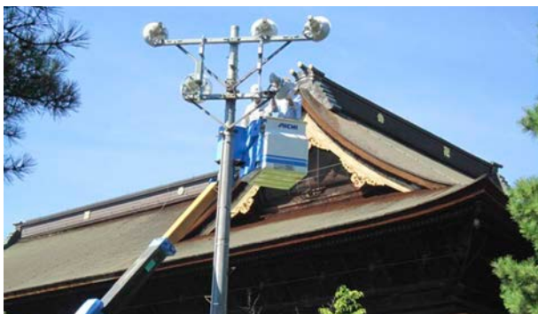
Electrical inspection at the Zenkoji Temple in Nagano City, Nagano Prefecture, performed jointly by the Electric Works Federation and the Chubu Electrical Safety Services Foundation.
