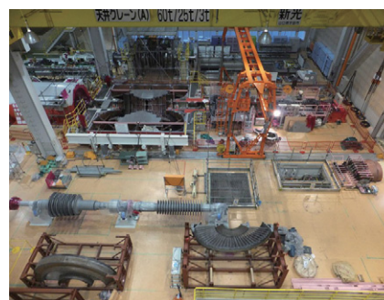
Regular inspection of the equipment
