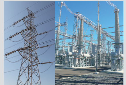
Transmission line tower and a substation
