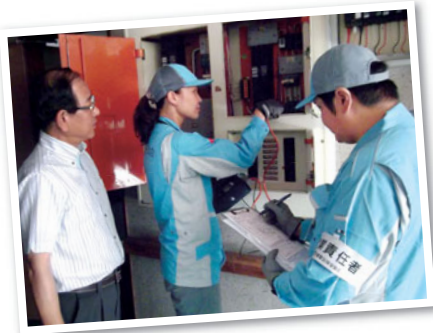
1 Checking of electrical facilities at elderly care centers (implemented by the Chubu Electrical Safety Services Foundation)
